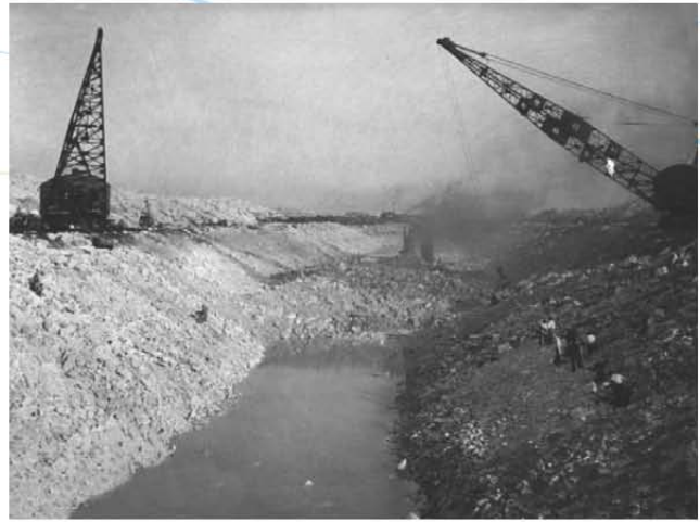
Digging the canal in Palos Park, Ill., in 1914. Pictured is the construction of the Calumet feeder to the drainage canal.
